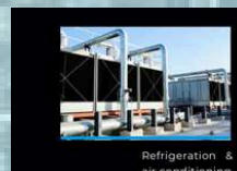
Refrigeration & air conditioning
