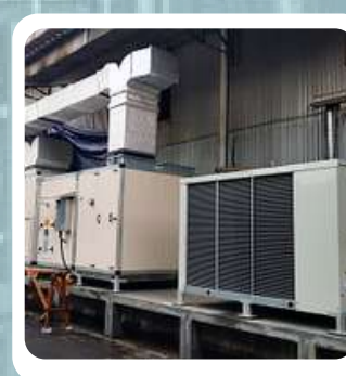
Air Handling Unit
